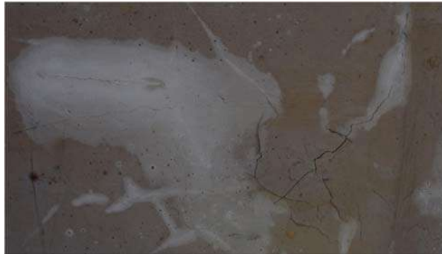
図4 Example of crack
